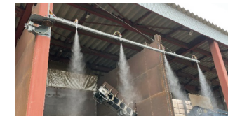
In-plant measures to control dust
